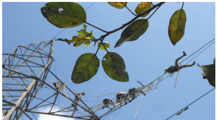
Contract workers carry out maintenance activity on the MSEDCL High Tension cables in a gravity defying act in the city. (By Ashok Dhamija)
